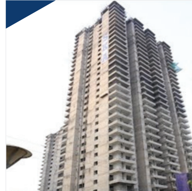
Client Name: SKA Group Project Name: SKA Divya
